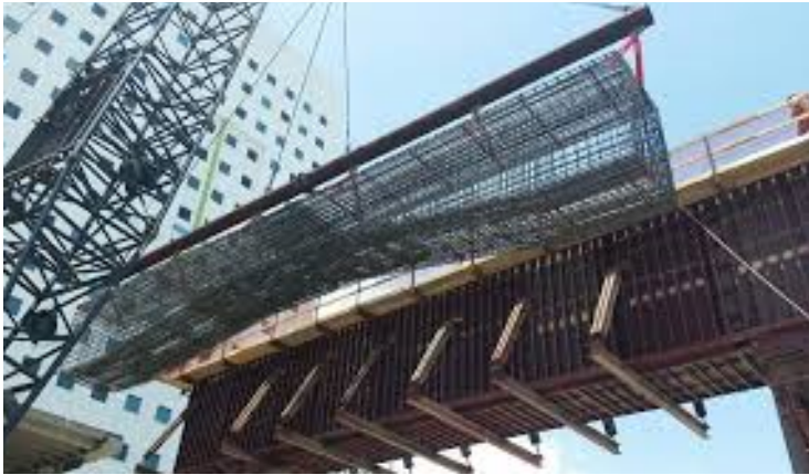
Pictured: Rebar cage suspended over project I-4 Ultimate Highway Expansion Project in FL prior to the accident
