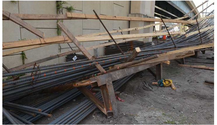
Pictured: The Same rebar cage after it collapsed.
